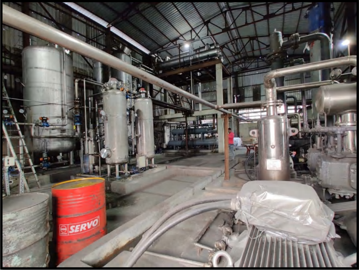
Photograph of the CO2 Plant
