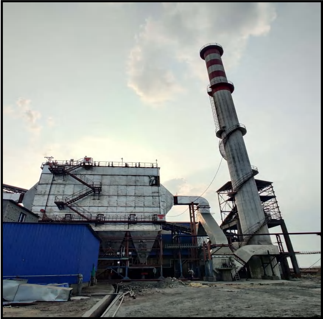
Photograph of the boiler stack with ESP
